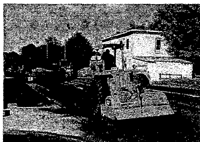
The Travel Mixer shown stabilizing existing asphalt road sub-base to 12" depth and 84" width.
